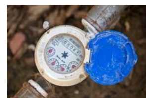
Water meter at a DP
