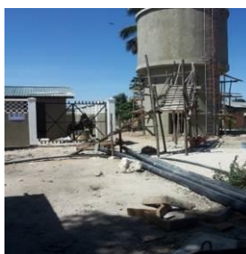
Storage Tank and Pumphouse at Yombodoya
